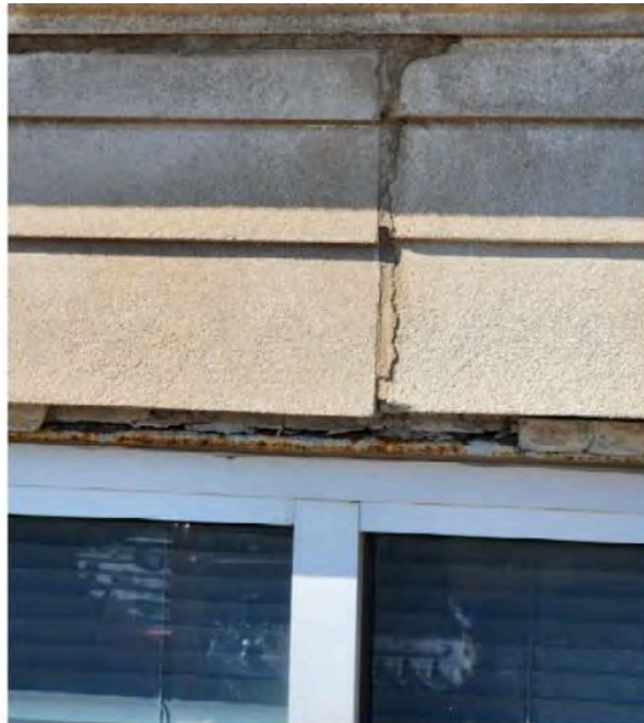
Corroded steel lintel with deteriorated/missing mortar fill at west façade.
